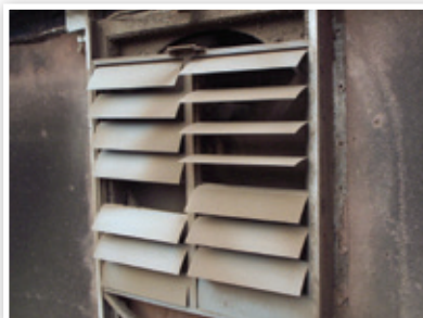
Broken flaps are a common maintenance fault
