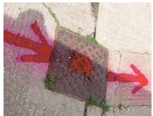
Drain cover painted red with flow direction arrows
