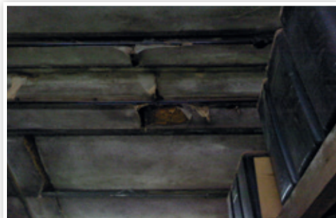
An example of poor roof insulation that is in need of replacement
