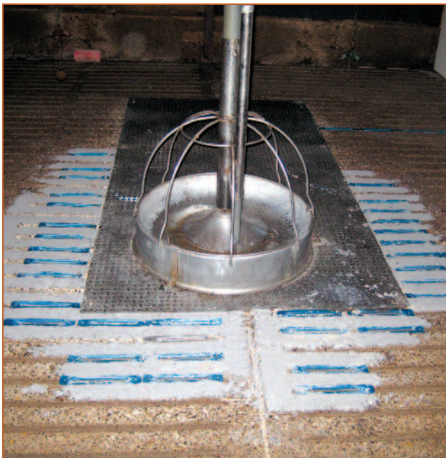
Repair of damage around feeder using a combination of granite/epoxy compound and slot reducers
